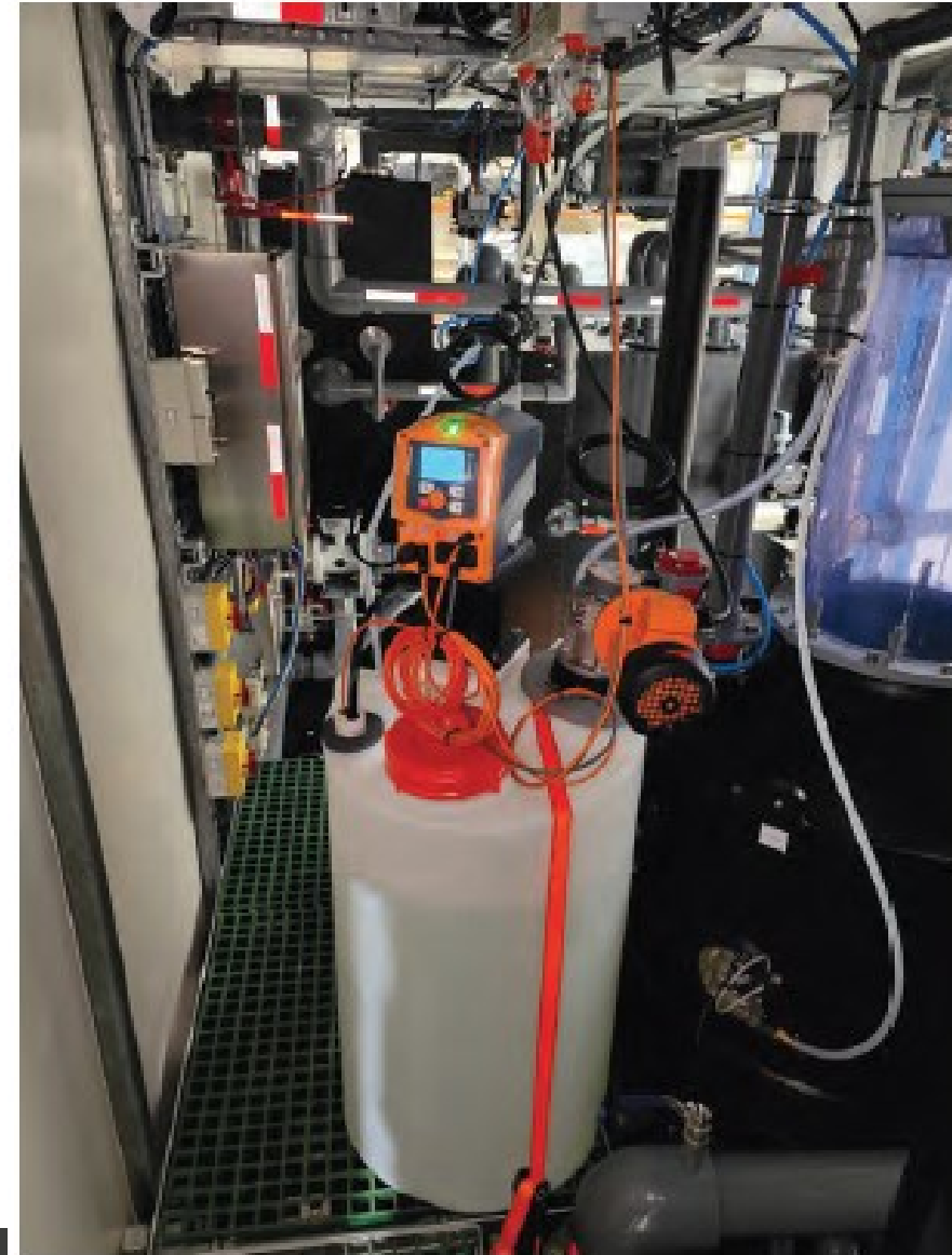
Figure 20: Dosing tank and pump
